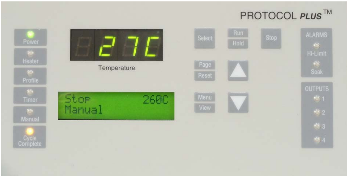
Close up view of controller
